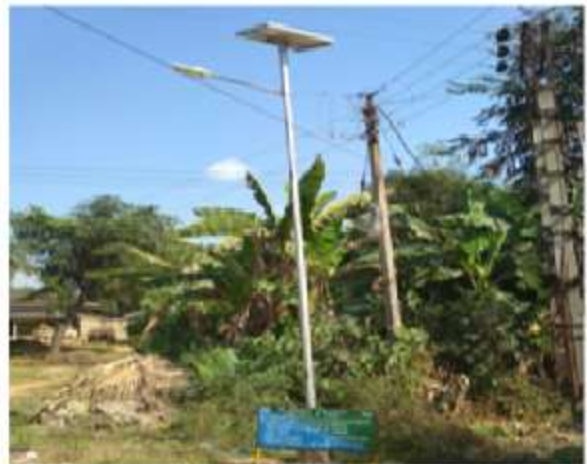
Installation of Solar Light under WBFBCP DMU:- Bankura North, FMU:- Sonamukhi, Beat- Hamirhatti, FMC-Ibuda GPS Location- N 23°16'34.2" E 87° 21'11.0"
