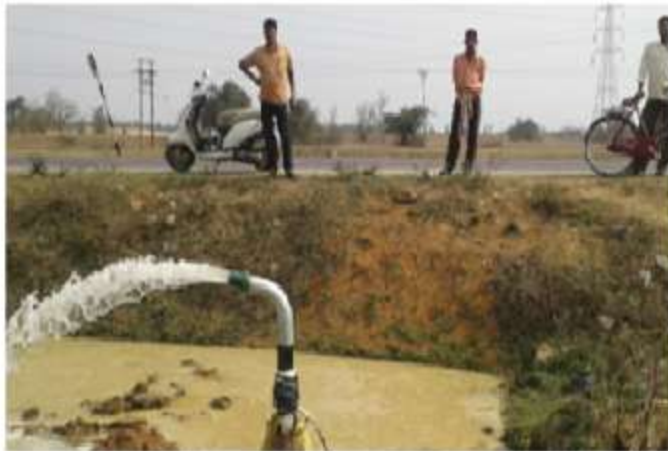
Deep Tube Well under WBFBCP DMU:- Bankura North, FMU:- Beliatare, Beat- Brindabapur, FMC-Shri Rampr Bhairabanga GPS Location- N 23°18' 56.80" E 86° 18' 48.31"
